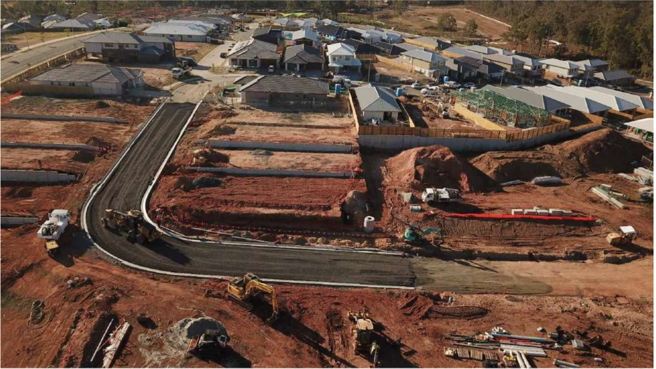
Photo 2: Aerial view of Stage 1 and Stage 2E – Housing and civil construction June 2019
